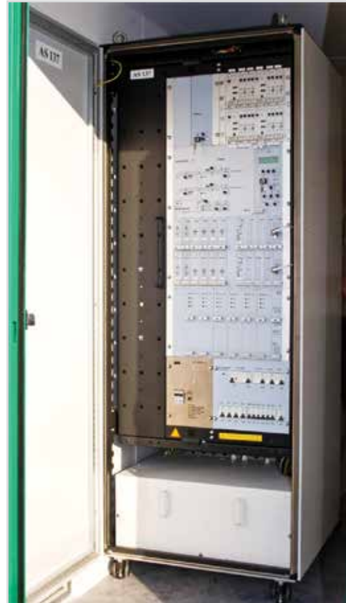
Power supply system with batteries integrated in a signalling system
