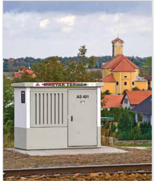
A UTB-M1 interlocking situated on the railway line of Raaberbahn in Kópháza
