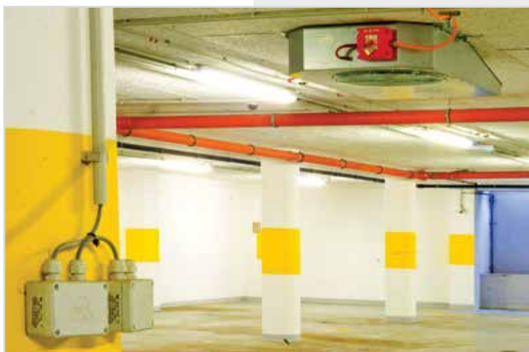
Integrated gas detector, fire detector and forced ventilation system in an underground parking lot
