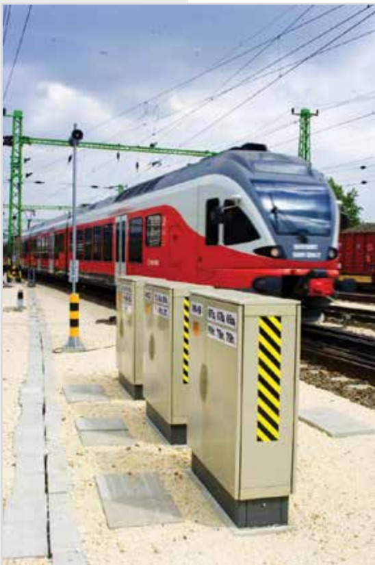
Control and switching cabinets for switch heating at mainline station Kelenföld
