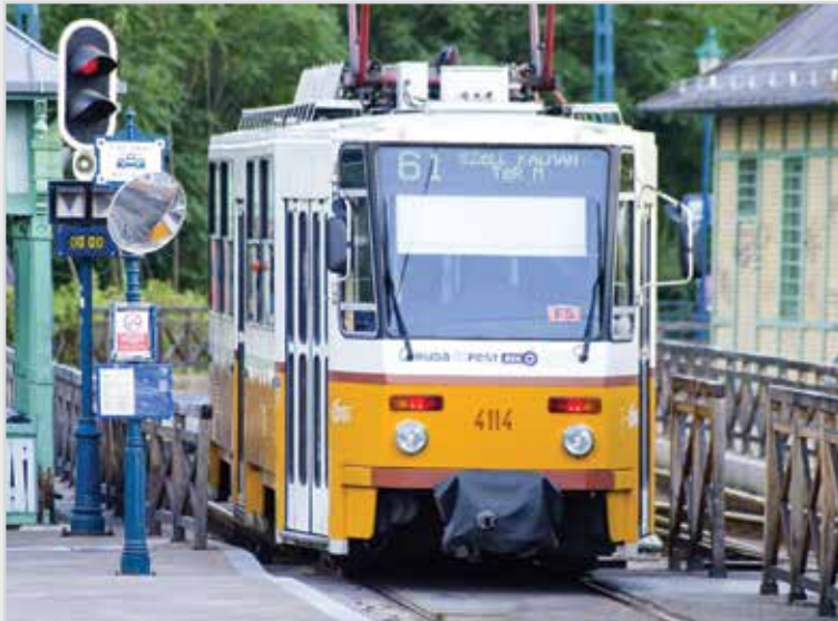
Tramway terminus signalling installed in heritage environment at Hűvösvölgy
