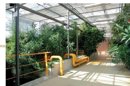
INSIDE AN ORGANICA TREATMENT PLANT
